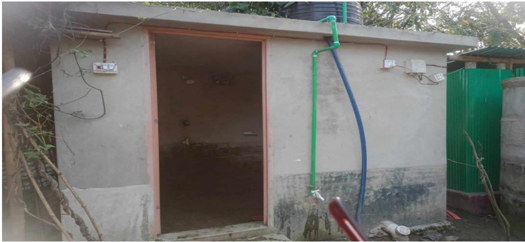
Figure 7: Project supported water and Hygiene facility
